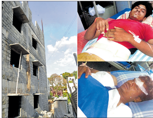
The building which crashed and the labourers Ram Singh of Manvi taluk of Raichur (above) and Ashok Kumar from the city (below) were seriously injured in the incident. DH PHOTOS
