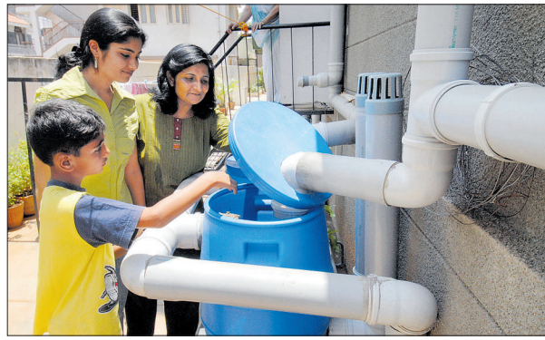
Properties without rainwater harvesting facility will have to pay an additional 25% on the bill for domestic connections and 50% for non-domestic connections for three months. The amount of fine doubles thereafter. DH FILE PHOTO
