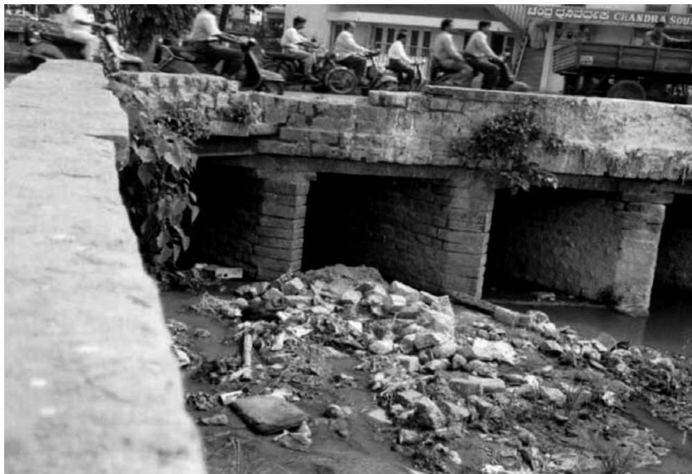
Plate 2.8: Reduced culvert capacity - dumping of solid waste and supports (Source: BWSSB)
