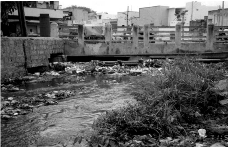
Plate 2.8: Stormwater flow hindrance from water pipes, solid waste, reduced culvert capacity
