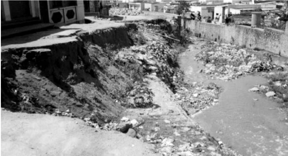
Plate 2.7: Bank erosion and instability due to modification in the floodplain
