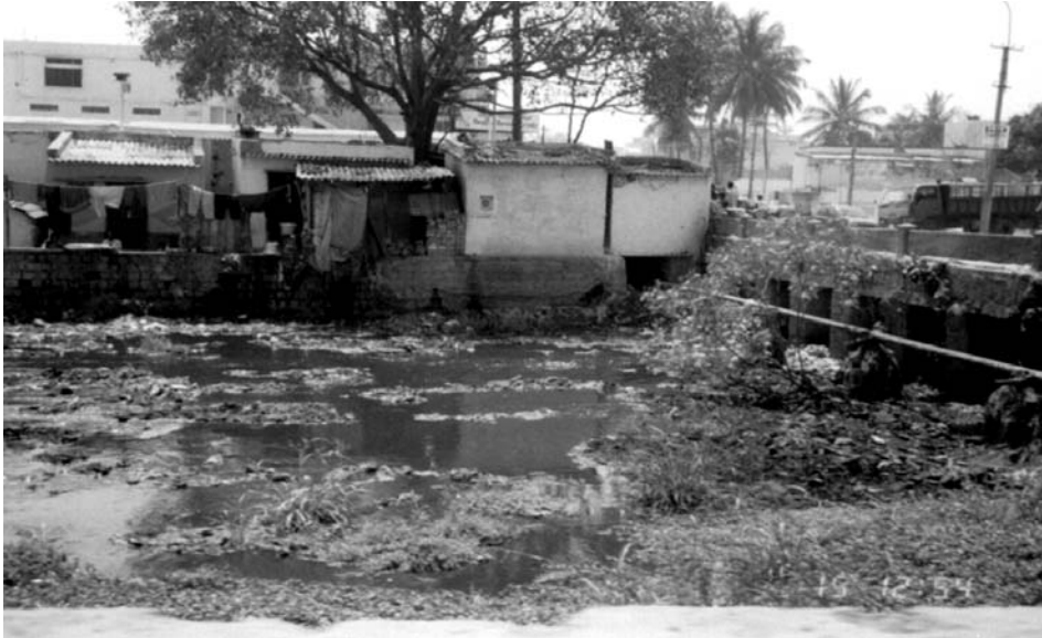
Plate 2.8: Reduced culvert capacity - dumping of solid waste and supports (Source: BWSSB)
