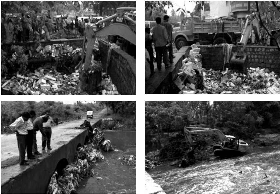
Plate 5.2: Removal of solid waste from the drain in KH Road, R.R. Nagar (Source: BMP)
