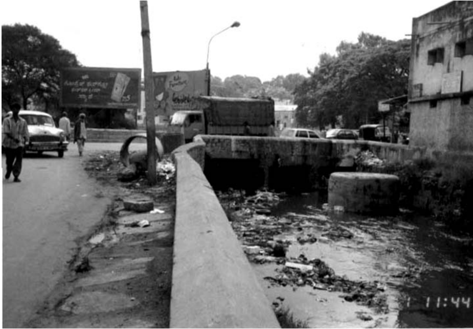
Plate 2.9: Sewer manhole, solid waste and under capacity road crossing
