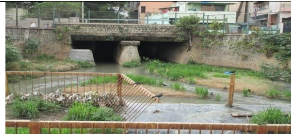
Sewage water flowing near the lake
