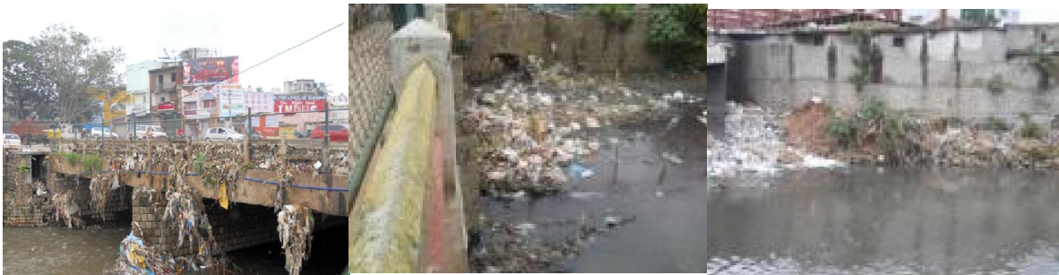
Fig 4: Drains littered with solid waste. Picture on left shows clear signs of flooding
