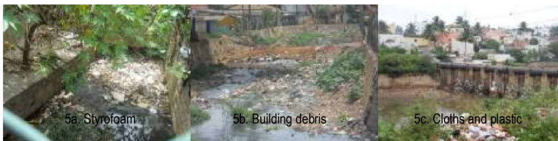
Fig 5: Solid wastes in storm water drains which can choke the water flow under peak conditions.
