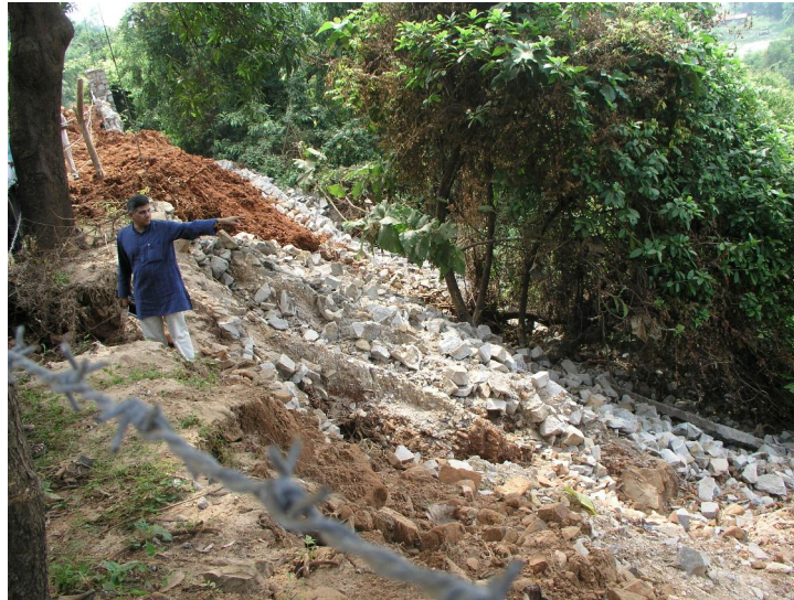
Figure 8: Landslide along NH-17, the slide material entering INS Kadamba Naval Base breaking through the compound wall
