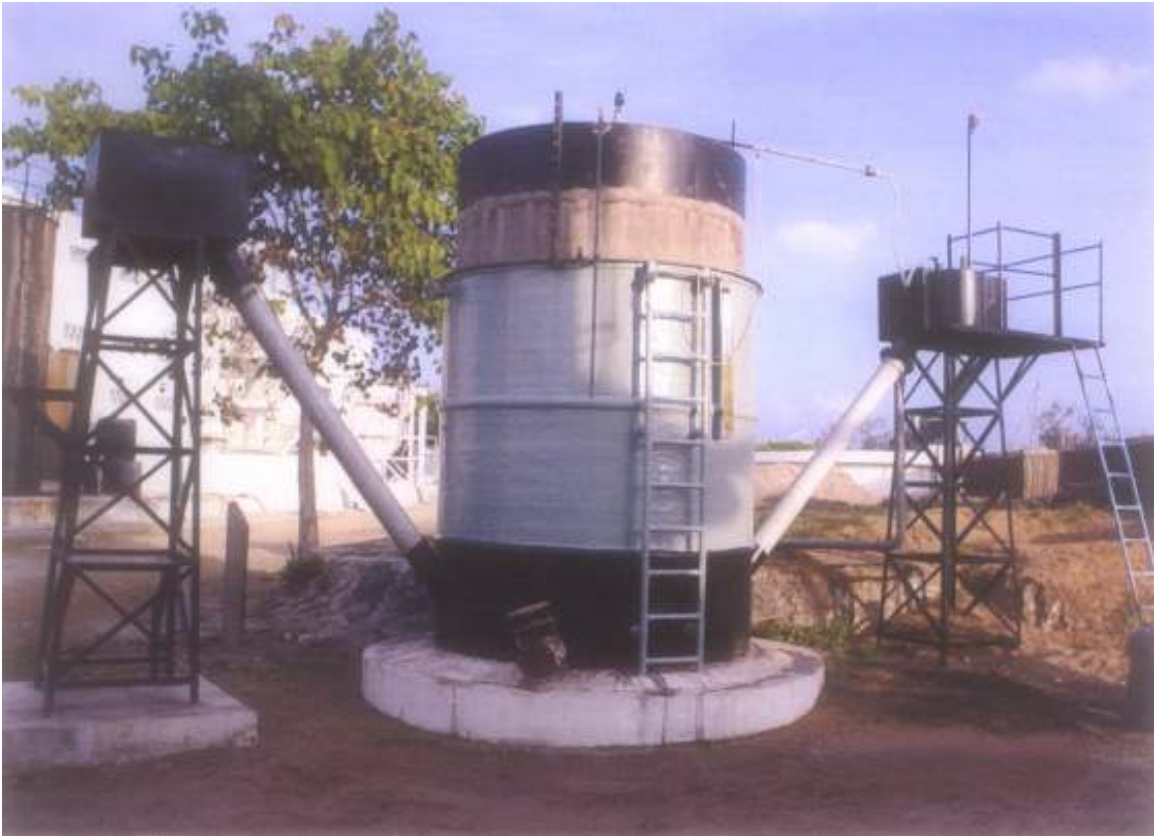
Figure –2 Bio-Gas Power Plant
