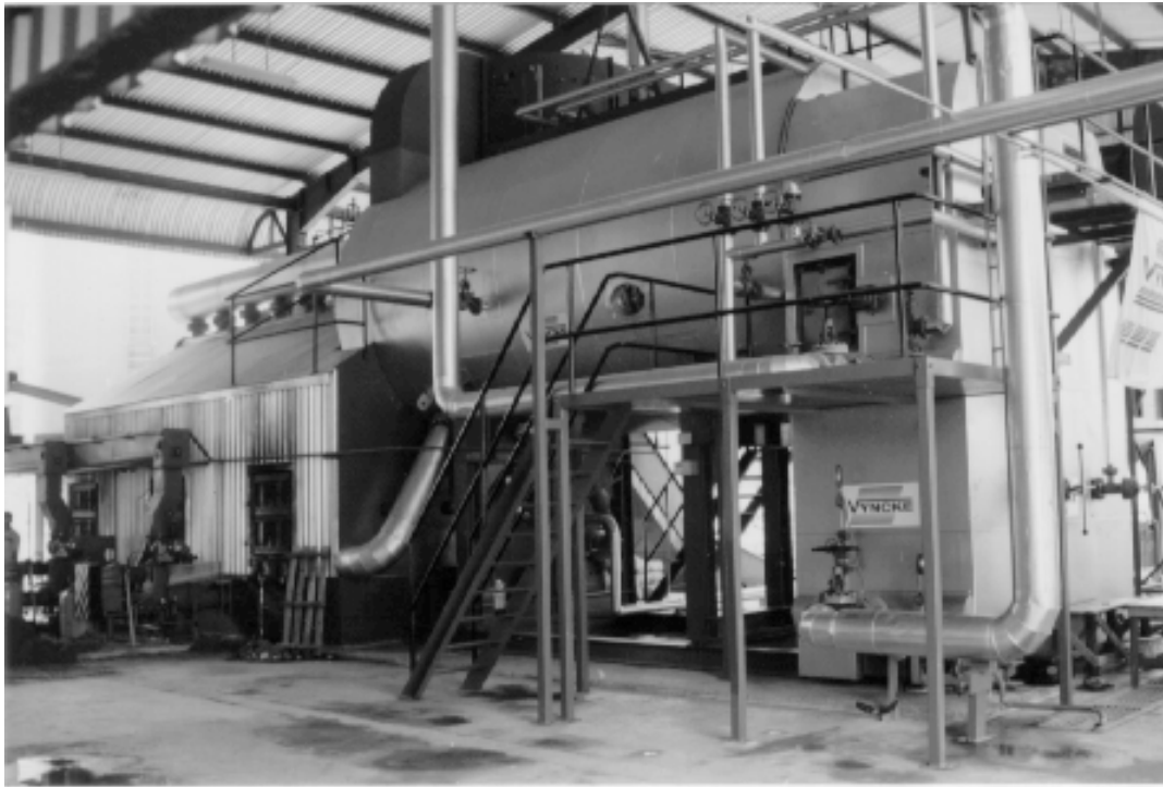
Furnace, boiler and superheater of the COGEN full-scale demonstration project at the IB Timber Industries Sdn Bhd wood processing plant
