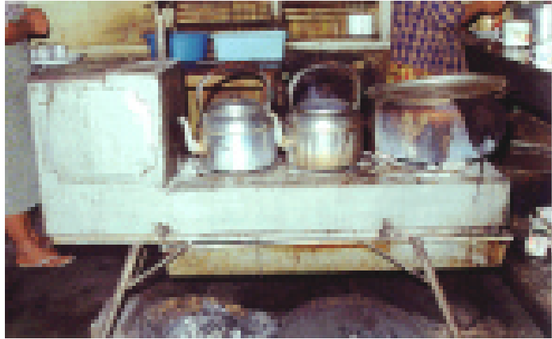
Figure 6.4 A boiler-type charcoal stoves used in teashop
