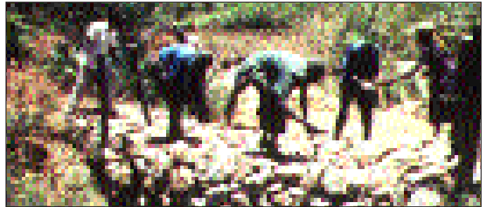
Check dams, such as this one being built in a gully in Kenya, can be used to trap sufficient sediment to give vegetation a chance to grow.
