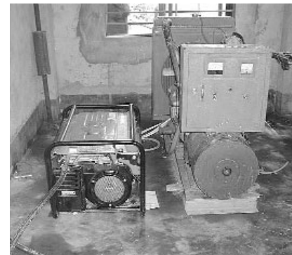
Figure 3.2 Biogas electricity generator at Faridpur Muslim Mission
