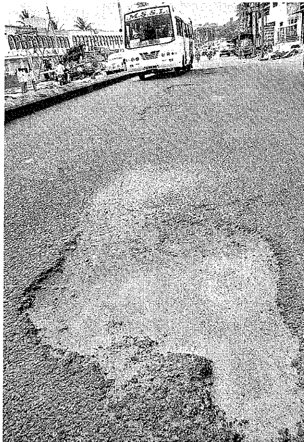
A CRATER THIS IS: The damaged Magadi Road which was developed under KMRP two months ago — PHOTO: K MURALI KUMAR
