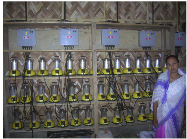
Fig. 2. View of a typical solar charging station.
