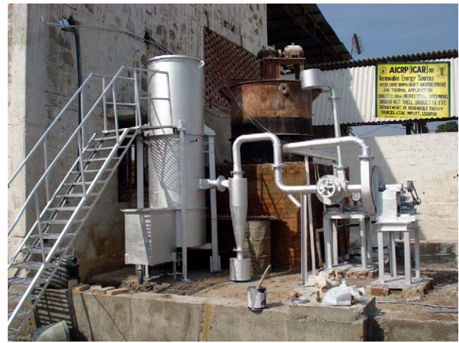
Fig. 10. Gasifier installed at M/s Phosphate India Pvt. Ltd., Udaipur.
