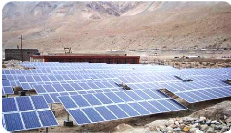
Fig. 4. A 100 kV solar power plant installed at Durbuk Block, Ladakh.
