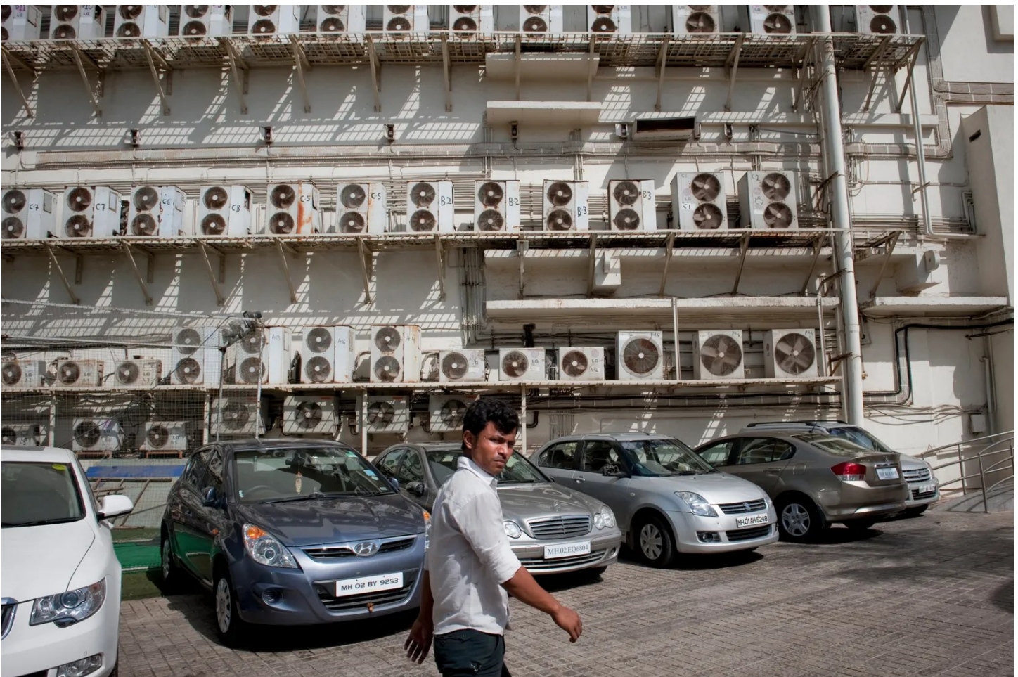
Air conditioning units installed outside of a shopping mall in Mumbai in May 2012. Chiara Goia—The New York Times/Redux
