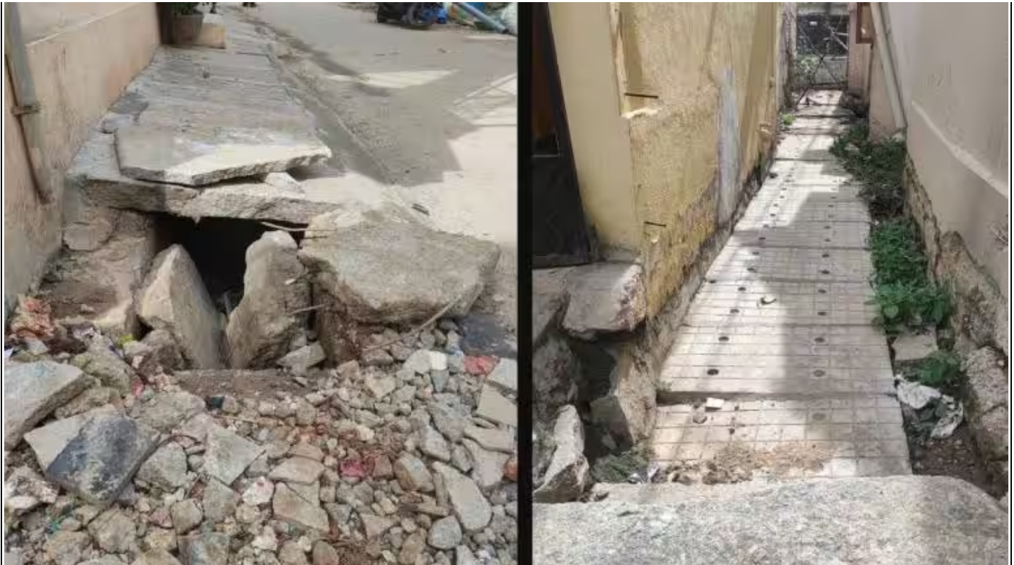
Stormwater drains in the area obstructed by debris or encroached by houses (Credit: Souptik)
