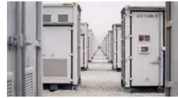
Significant growth opportunities in Indian Battery Energy Storage...
