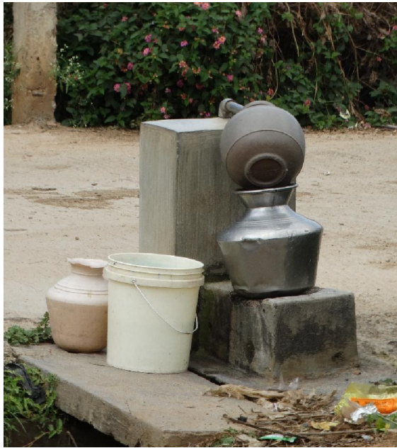
Figure 7: Common tap facility
