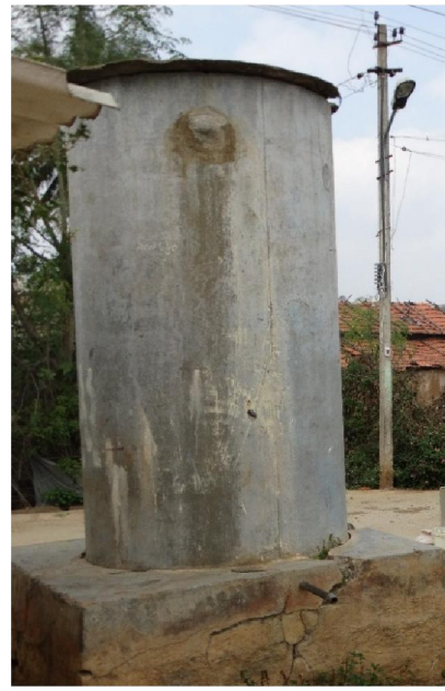
Figure 8: Community water storage tank
