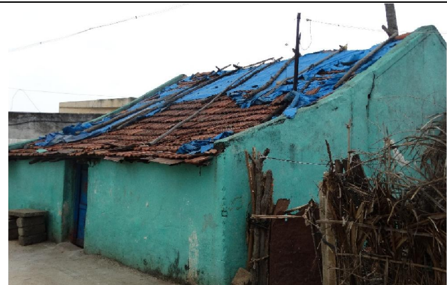
House with mud walls and fragile roof
