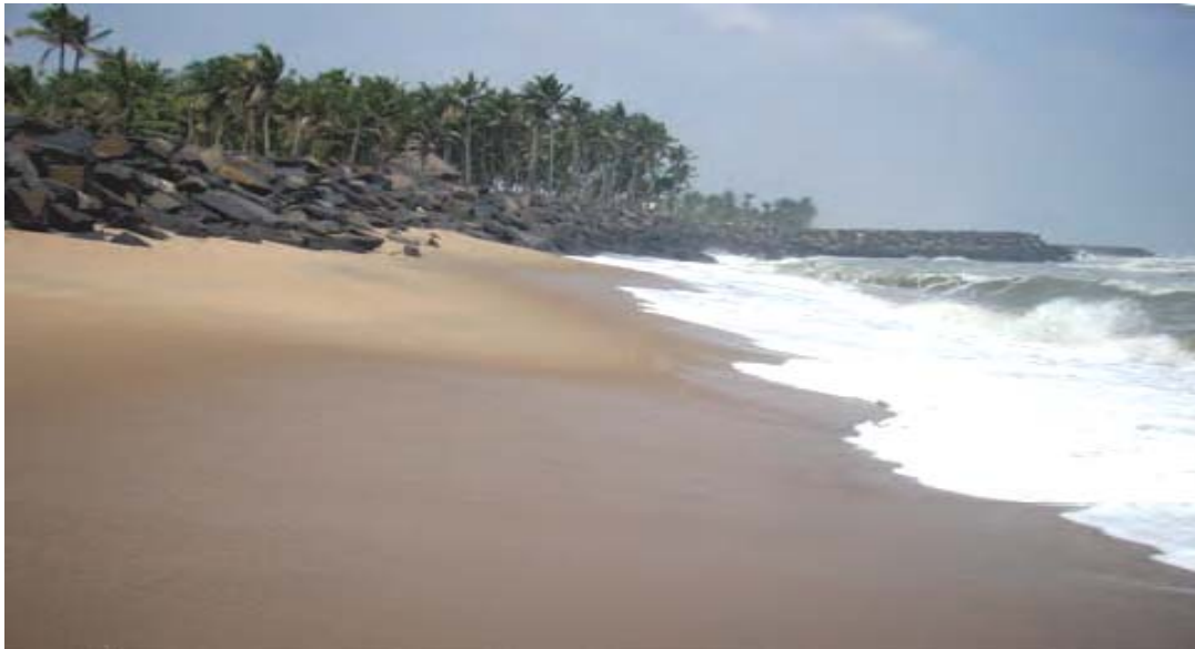
Fig. 3.4: A stone wall protected beach showing subsidence and lack of vegetation
