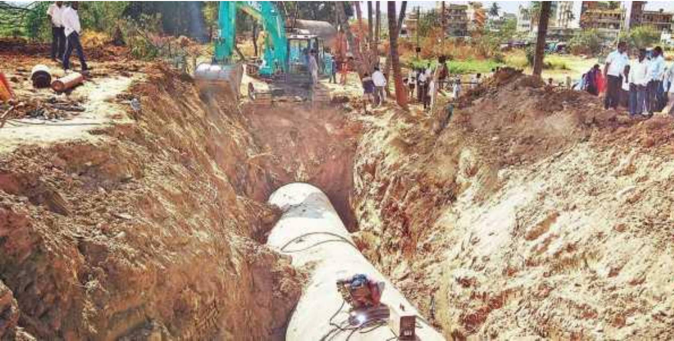
Work on Koramangala Challaghatta (KC) Valley project in progress at Kolar | Express
