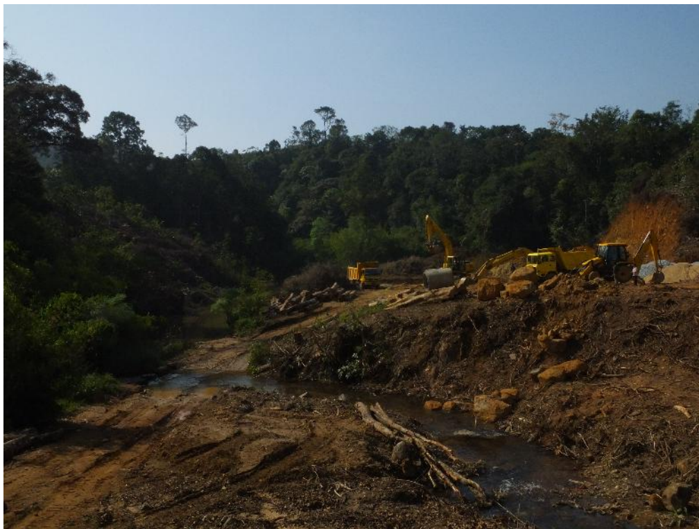
Earthmoving work underway at one of the sites of the Yettinahole project. Credit: Meghna Krishnadas
