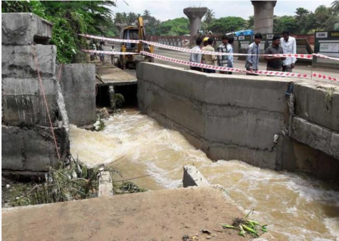
BBMP has created a temporary pathway at Vrishabhavathi valley on Mysuru Road to enable flow of water overflowing from the Dubasipalya lake. DH Photo
