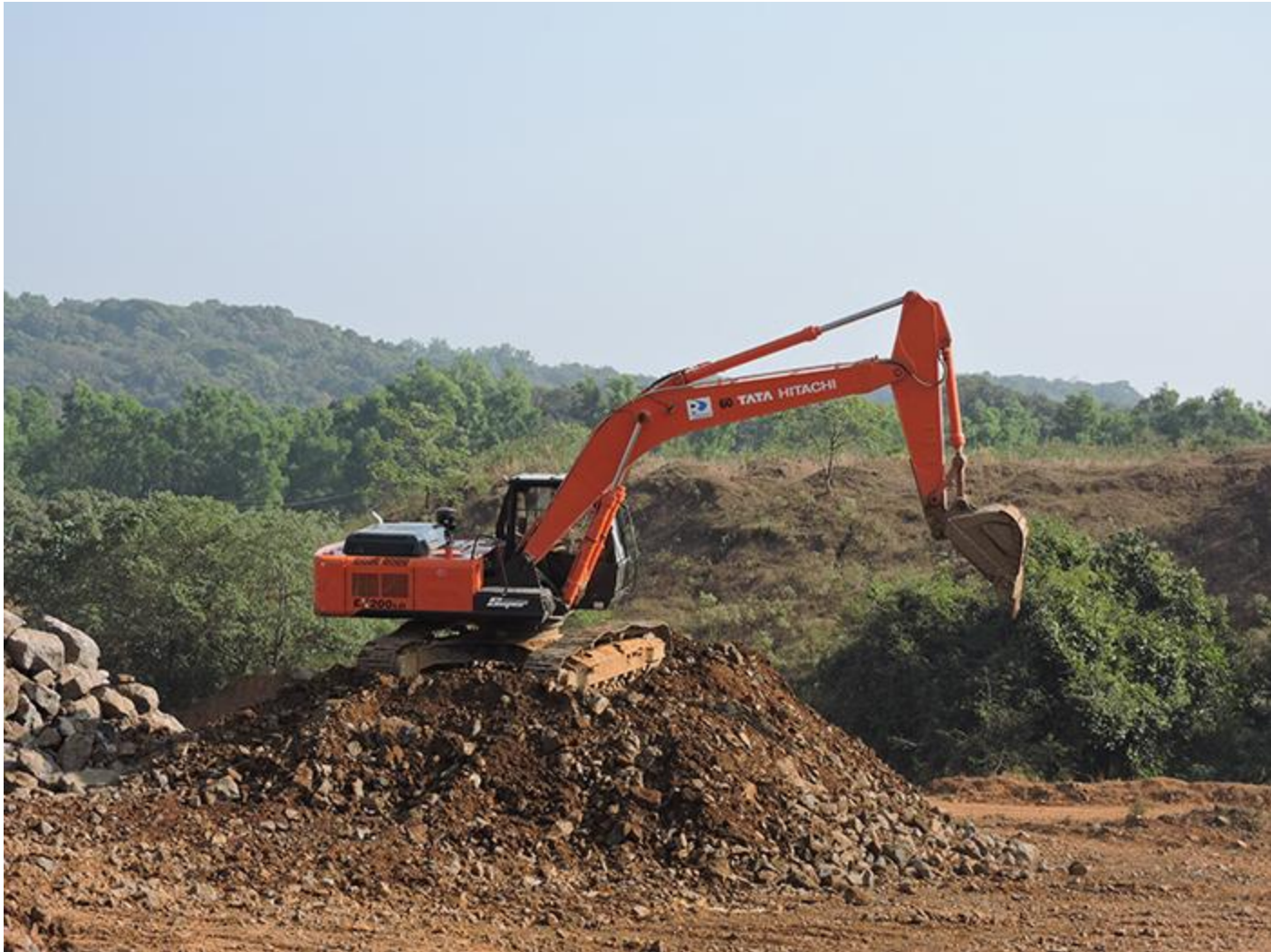
Construction work in the catchment area has affected the river.
