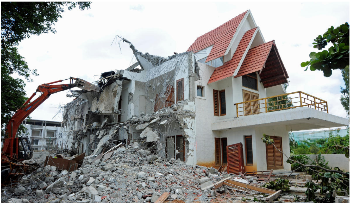
Demolition of a villa at Shubh Enclave in Kasavanahalli, in 2016. Encroachment of storm water drain had resulted in severe flooding in this area. (DH Photo/Ranju P)
