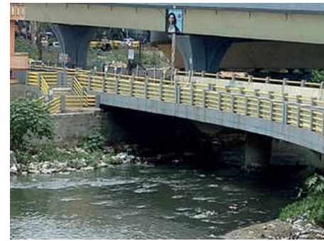
It is feared that blocking or narrowing down of this SWD could inundate parts of Indiranagar, Domlur and Jogupalya in the event of a heavy downpour.
