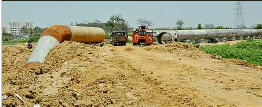
A mud road being laid through the Varthur Lake for laying a pipeline. DH FILE PHOTO
